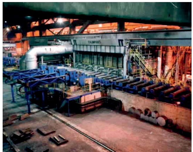
Figure 4.8. Walking beam furnace.
