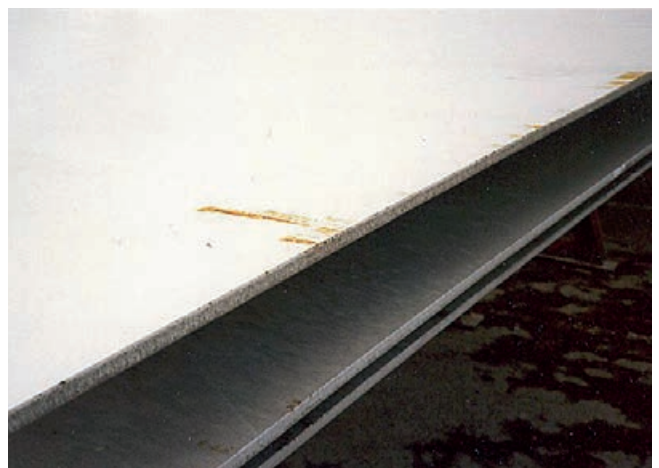
Figure 12:2. Staining caused by iron contamination from truck forks.
