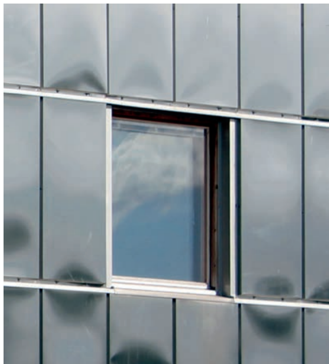
Figure 8:2. Austenitic stainless façade which has buckled under intense sunlight. Unless this is desired as an architectural feature, a duplex or ferritic grade with lower thermal expansion may be preferred.
