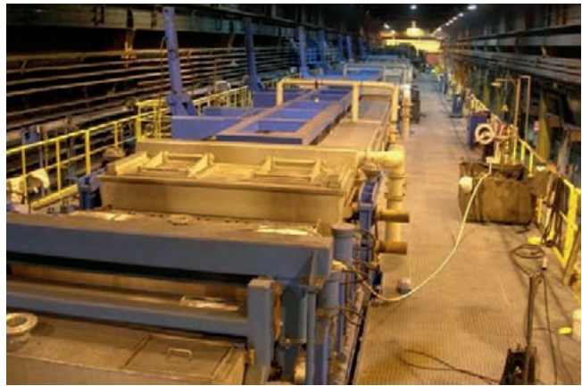
Figure 4:11. Mixed-acid pickling line.
