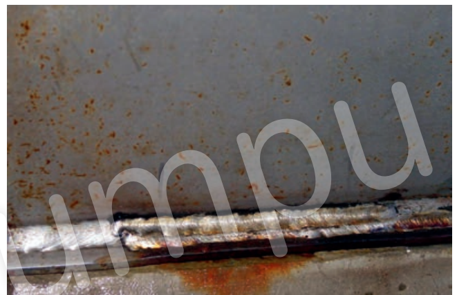
Figure 11:3. Lack of fusion in welds can cause corrosion attack.
