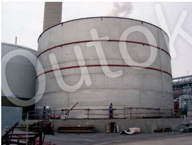
Figure 9:17. White liquor tank in duplex LDX 2101®, where corrosion resistance and strength of this grade is utilized.
