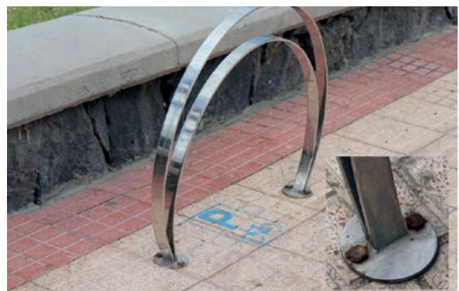
Figure 6:18. Bicycle parking on Tenerife, Canary Islands, 100 m from the Atlantic Ocean. Galvanic corrosion on galvanized bolts.
